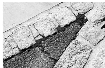
10.41 Below: Example of a cracked pavement within an acute angle.
