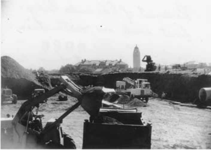
FIGURE 1.4. Construction of Edwards Building, Stanford Medical School. The medical school moved to the main campus at Palo Alto, ca. 1958. Image from Arthur Kornberg Papers, Stanford University Archives, SC 359, box 31. Reproduced with permission, Department of Special Collections, Stanford University Libraries, Stanford University.
