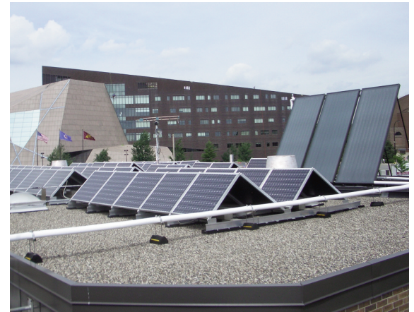
Solar PV and solar hot water arrays on Fire Station No. 19 Photo Credit: City of Minneapolis
