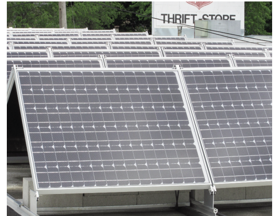
The Solar PV array atop of Quality Coaches
